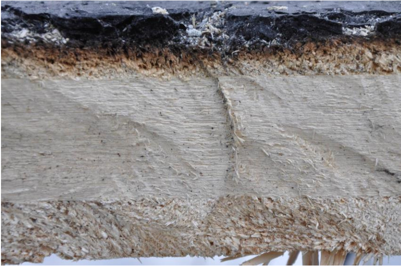
Fig. 1: cross-section of an 80 mm CLT element, originally clad with fire protection plasterboard, after a large-scale fire test
